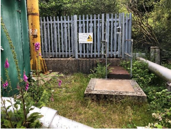
Photo Collection 1: Views of Diversion Culvert Sumps including Overflow discharge into Nant Gwylan, north of the site NGR - SH 69274 38321
